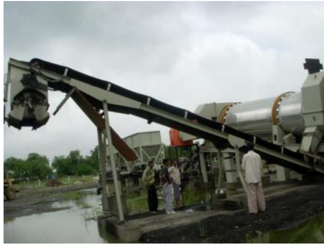
Fig. Load Out Conveyor
