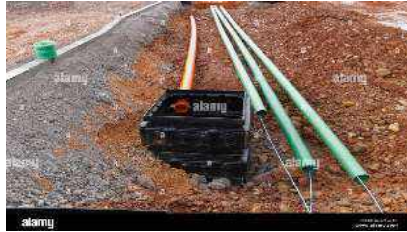
An access chamber (or manhole) is a structure designed to allow access to an underground service, such as a stormwater pipe or a sewer.
