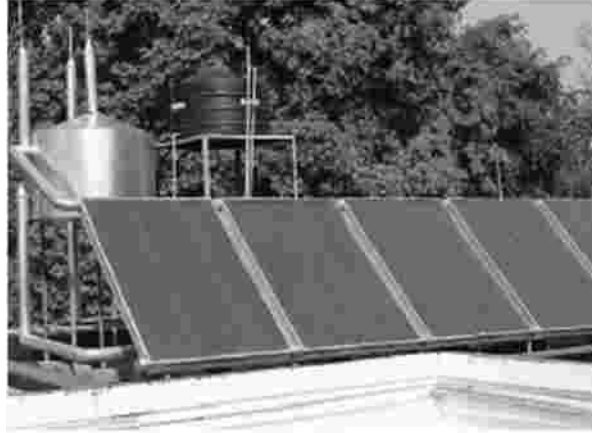
Figure 5.18 Solar water heater
